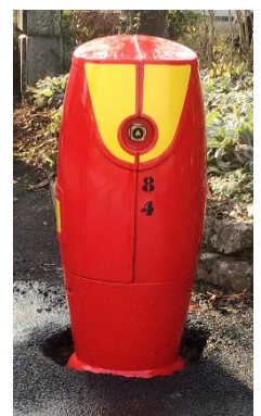
Figure 5 : Poteau incendie DN150.
